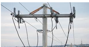
Distribution Power Poles
